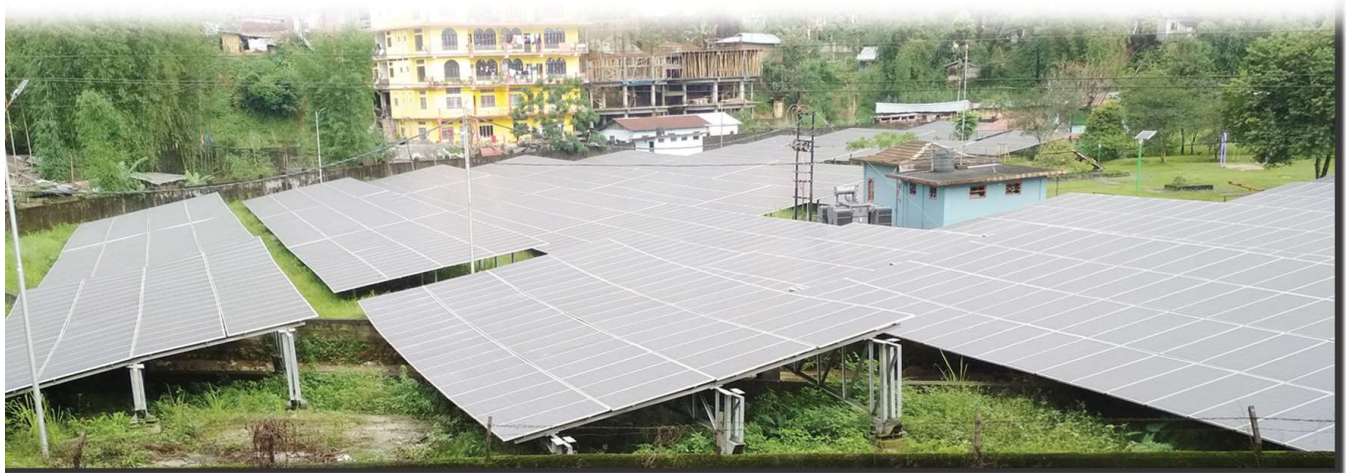
1 MW Solar PV Power Plant, at Energy Awareness Park, Itanagar
